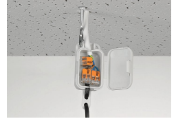
Pendant light connection in a suspended ceiling
